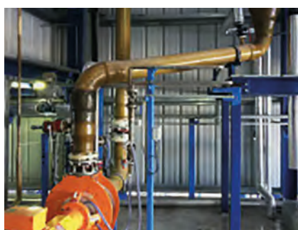
Circulation Pipe of Calcium Chloride Evaporator
