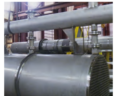
Heating Chamber for a Potassium Chloride Crystalliser
