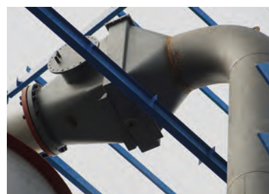
Droplet Separator in Vapour Duct
