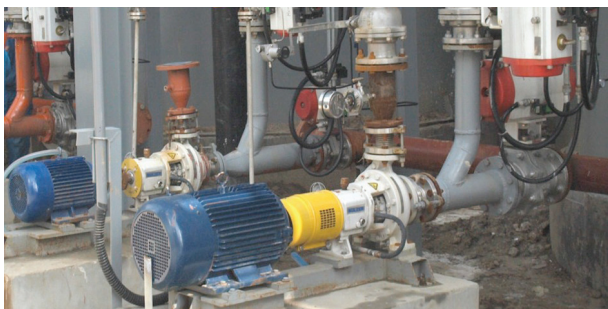
Pumping Station for Chemical Additives
