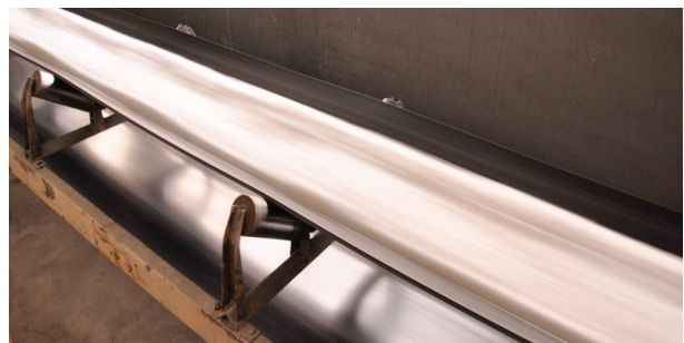
Dry Salt Conveying
